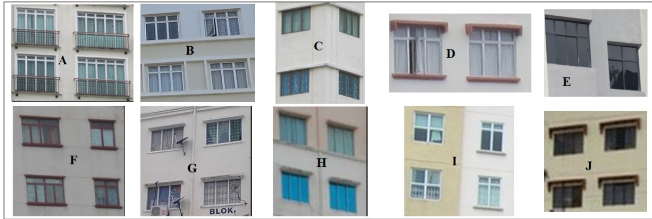
Figure 5. Lack of external shading controls on the facades of case studies: (A)Pulai View, (B)Kipark, (C)Danga View, (D)Kolej Perdana, (E)Mewah View, (F)Skudai Parade, (G)Pangsapuri Jasa, (H)Nusa Perdana, (I)Lake View Suite, (J)Flat Cempaka
