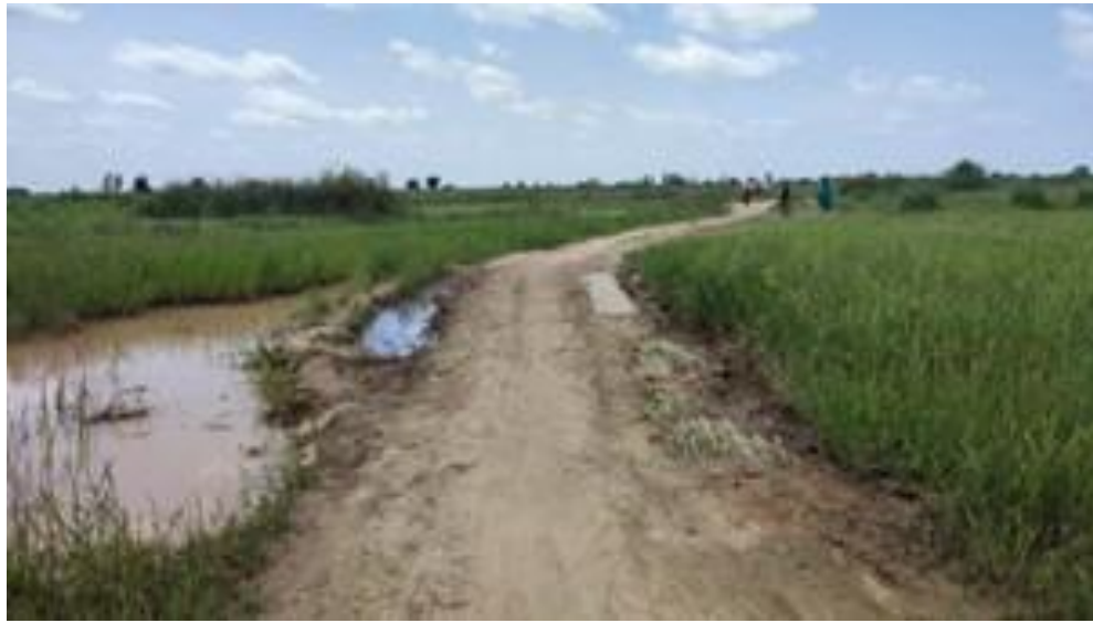
Figure 10 Use of Sandbags to augment potholes on the road at low levels(Authors' Fieldwork 2023)
