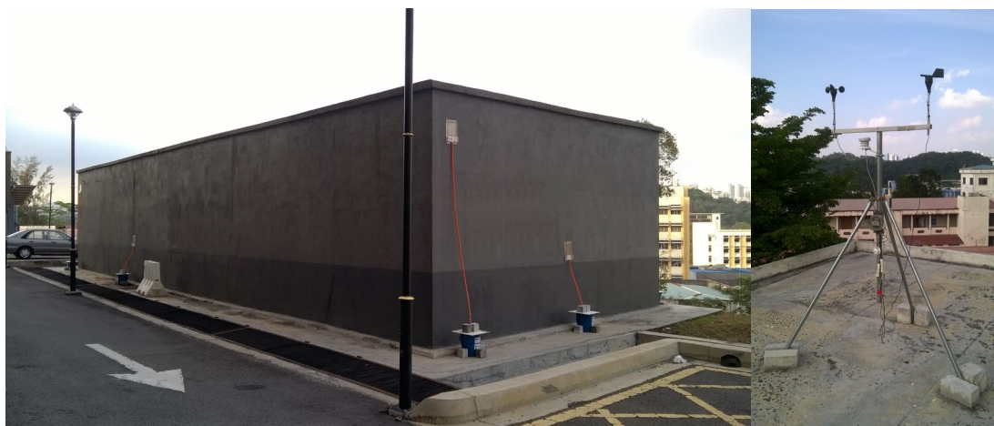
Figure 13 The pilot building and position of the WDR gauges on the facades (a) South view (b) Meteorological mast on the roof of the building at the parking area.
