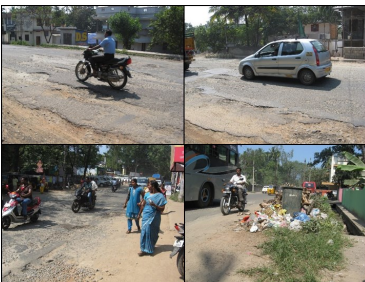
Figure 5 Dilapidated Road Conditions of NH-47
